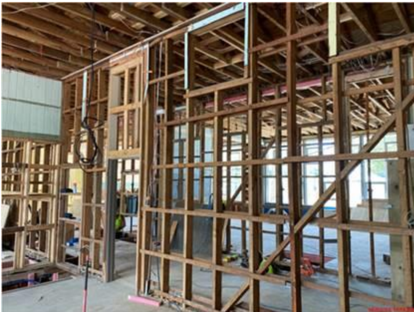
Photo 1 – Looking from Raumati through to Kauwhanga (double classroom) which looks out to Hohiria Road
